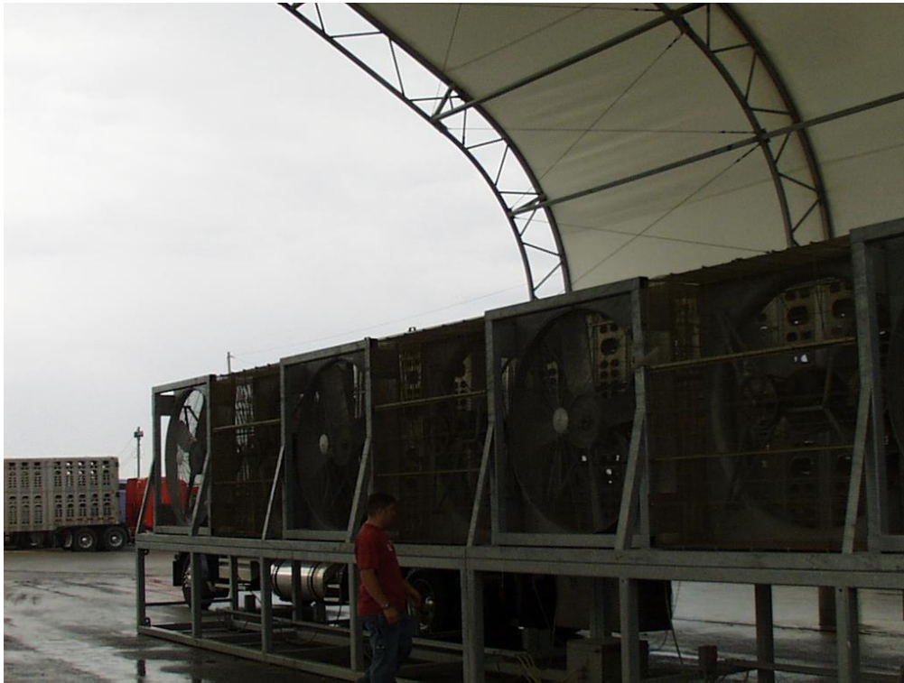
Figure 5a. Canopy and bank of cooling fans in waiting area at the plant
