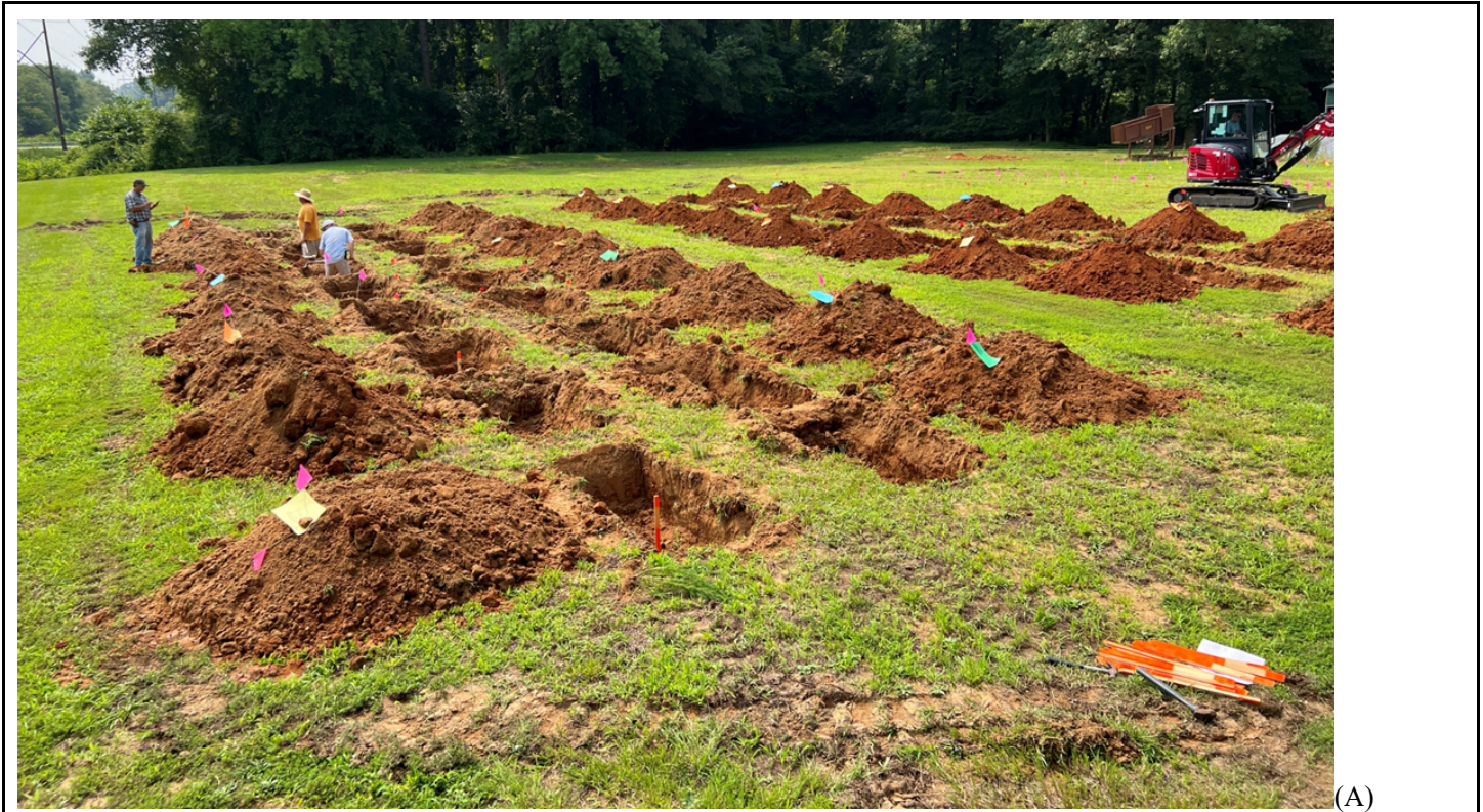
Figure 1. Experimental site after excavating the individual plots and before carbon material placement, and (B) tabular format showing experimental design
